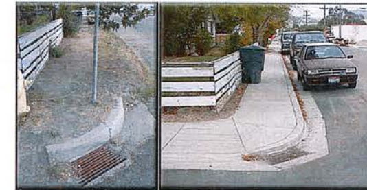
New sidewalks, curb and gutter were built with the Roosevelt TIF District
