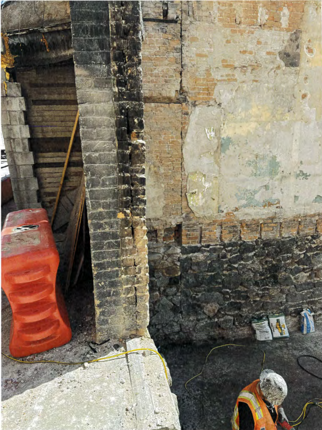
Photo 2 - Close-up of the exposed masonry at the cold joint and wall interface.
