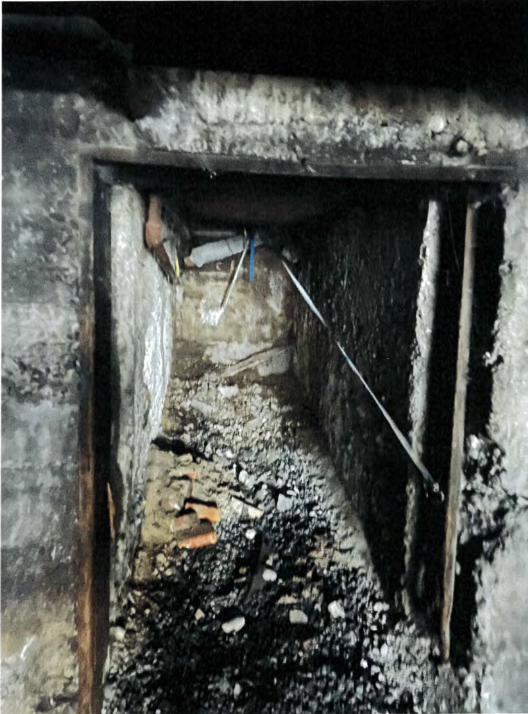
Photo 1 - Existing coal-chute void discovered beneath the sidewalk.
